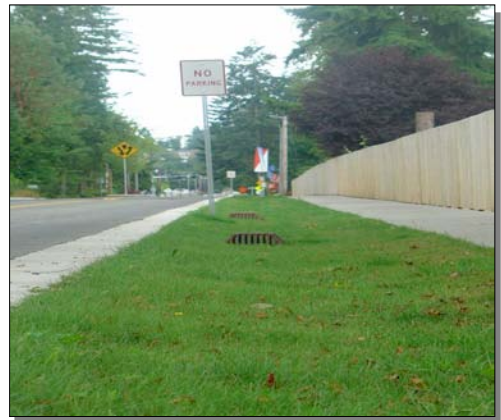
Caldart Avenue low-impact storm water drainage
